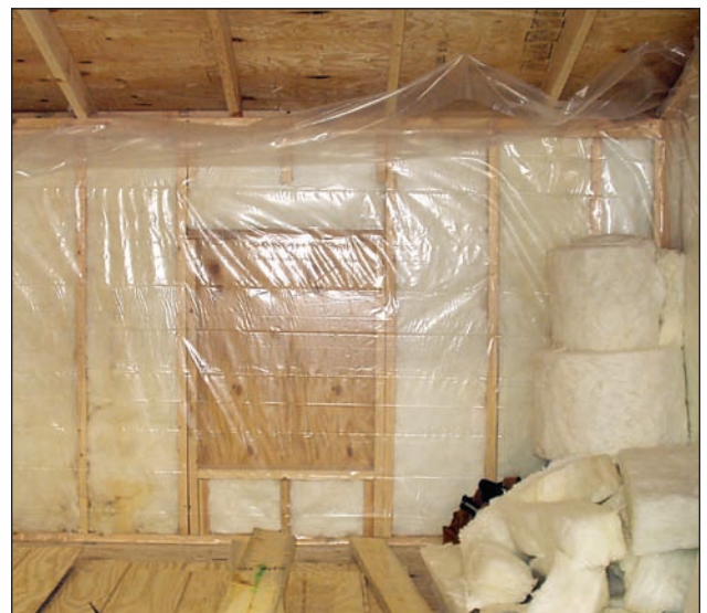
Figure 1: A plastic vapor barrier was used between the inside wall sheathing and wall studs.
